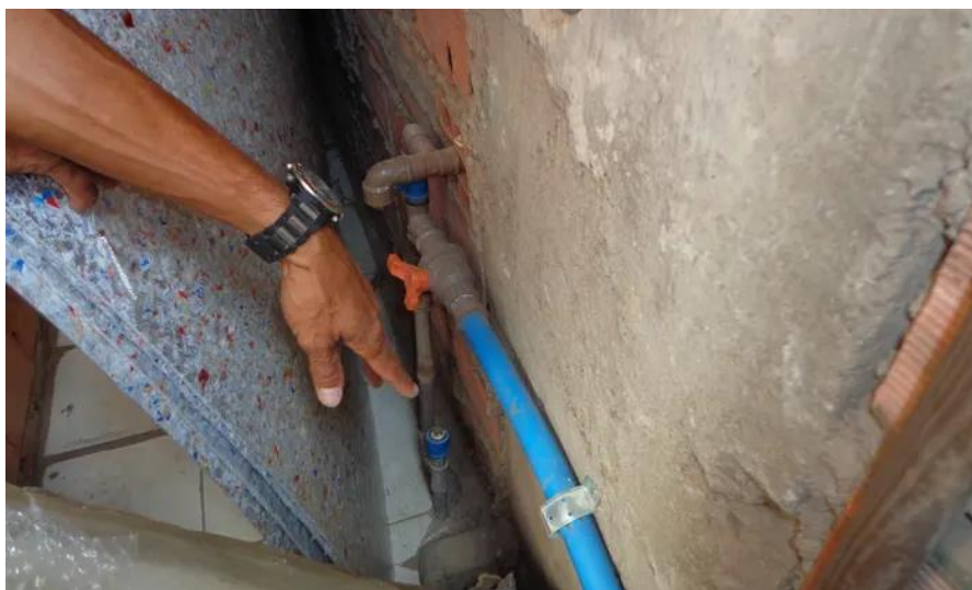
This PVC pipe was responsible for delivering water to the 2500 residents of the Favela de Mohino
